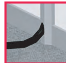
HIDDEN VENUE MAINS CABLE - PER BLOCK
